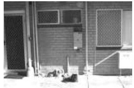
Typical water heater installation that will require an exemption
