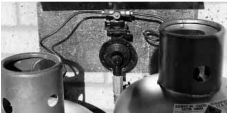
View of twin stage regulator fitted with a pressure test point and protected by a weather shield
