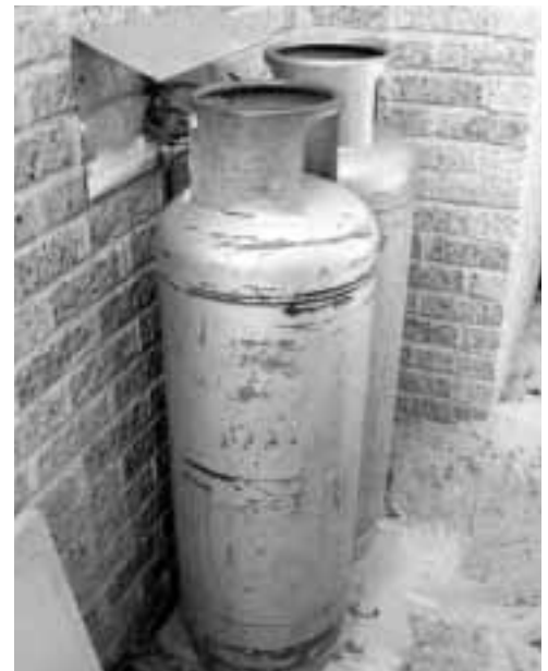
LPG cylinders correctly mounted on a firm base
