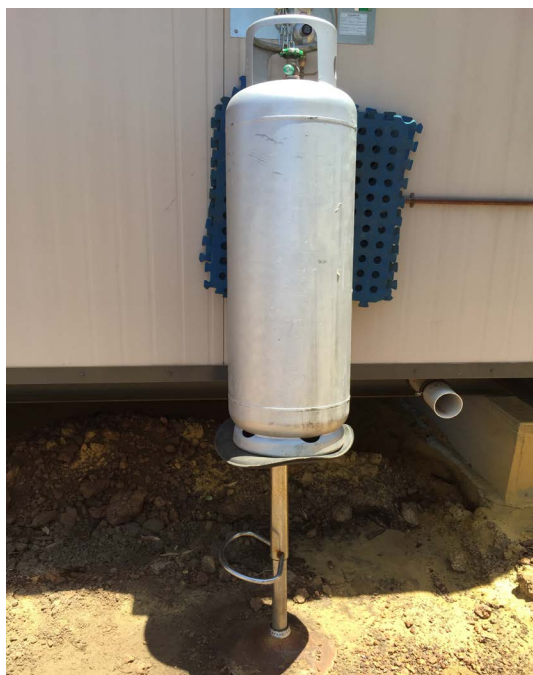
45Kg LP Gas cylinder installed on a bar stool
