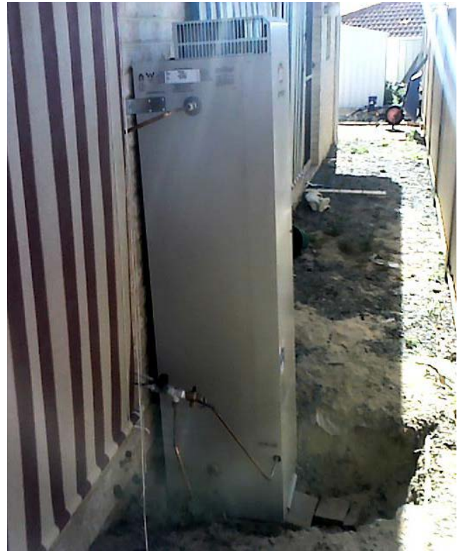
Gas hot water system installed in a hole
