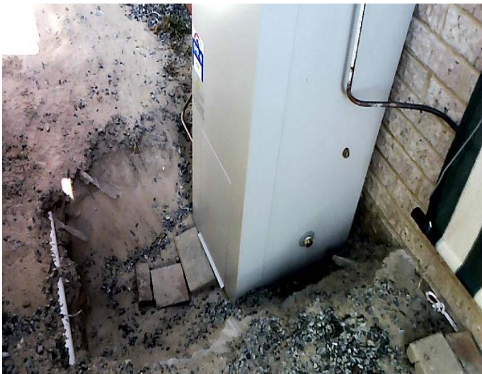
Gas hot water system installed in a hole
