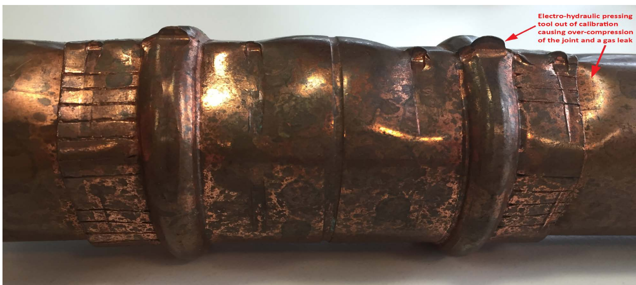
Over compression due to the electr-hydraulic pressing tool being out of calibration
