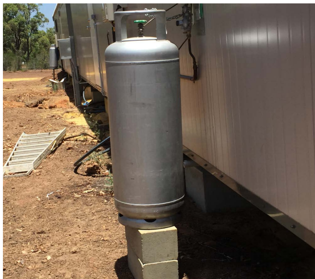
45Kg LP Gas cylinder installed on 'concrete breeze' blocks
