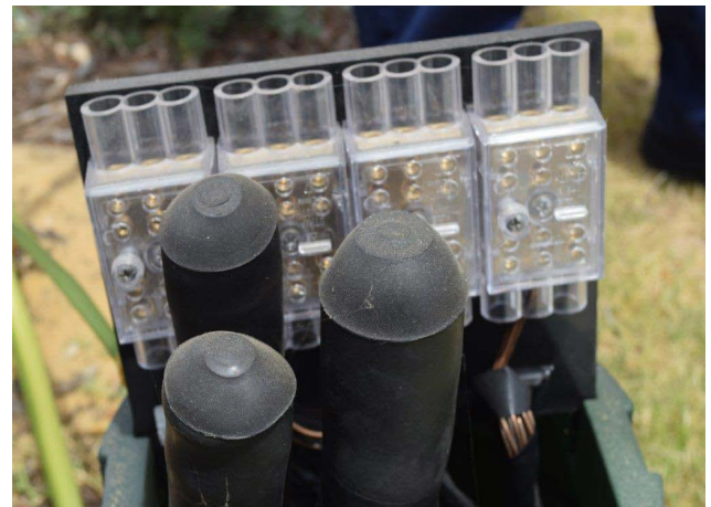
The three underground low voltage cable cores that had been made off at different lengths within the Western Power pillar
