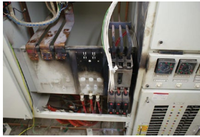
Switchboard showing the arc marks where the flashover occurred
