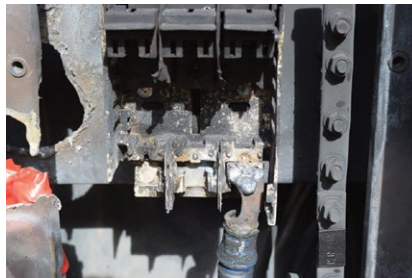
Arc marks and holes within the metallic structure of the switchboard attributed to the flashover
