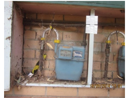
Typical old sub-meter
