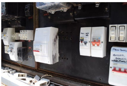
Main switchboard showing the Clipsal load centre with arc marks from the flashover
