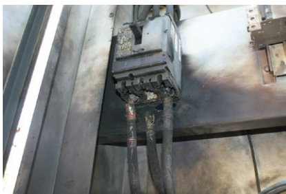
Arc marks surrounding the unprotected incoming main entering the main switch
