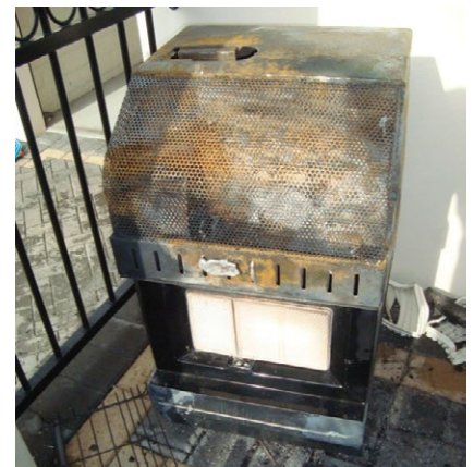
Damage to gas space heater
