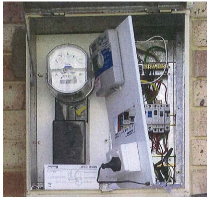
The 240 volt double socket outlet mounted on the front of the escutcheon plate of the main switchboard
