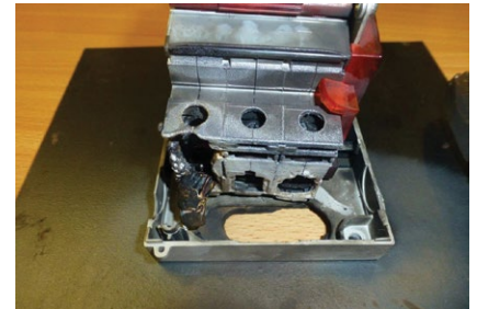
The melted metallic part of the line side of the installation's main switch
