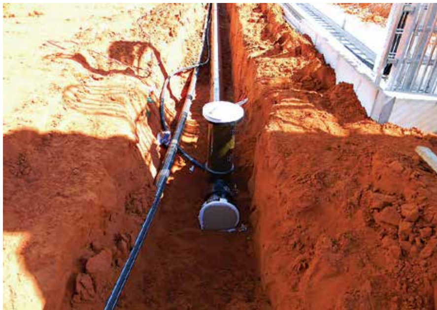
Underground GRE to above ground steel pipeline transition
