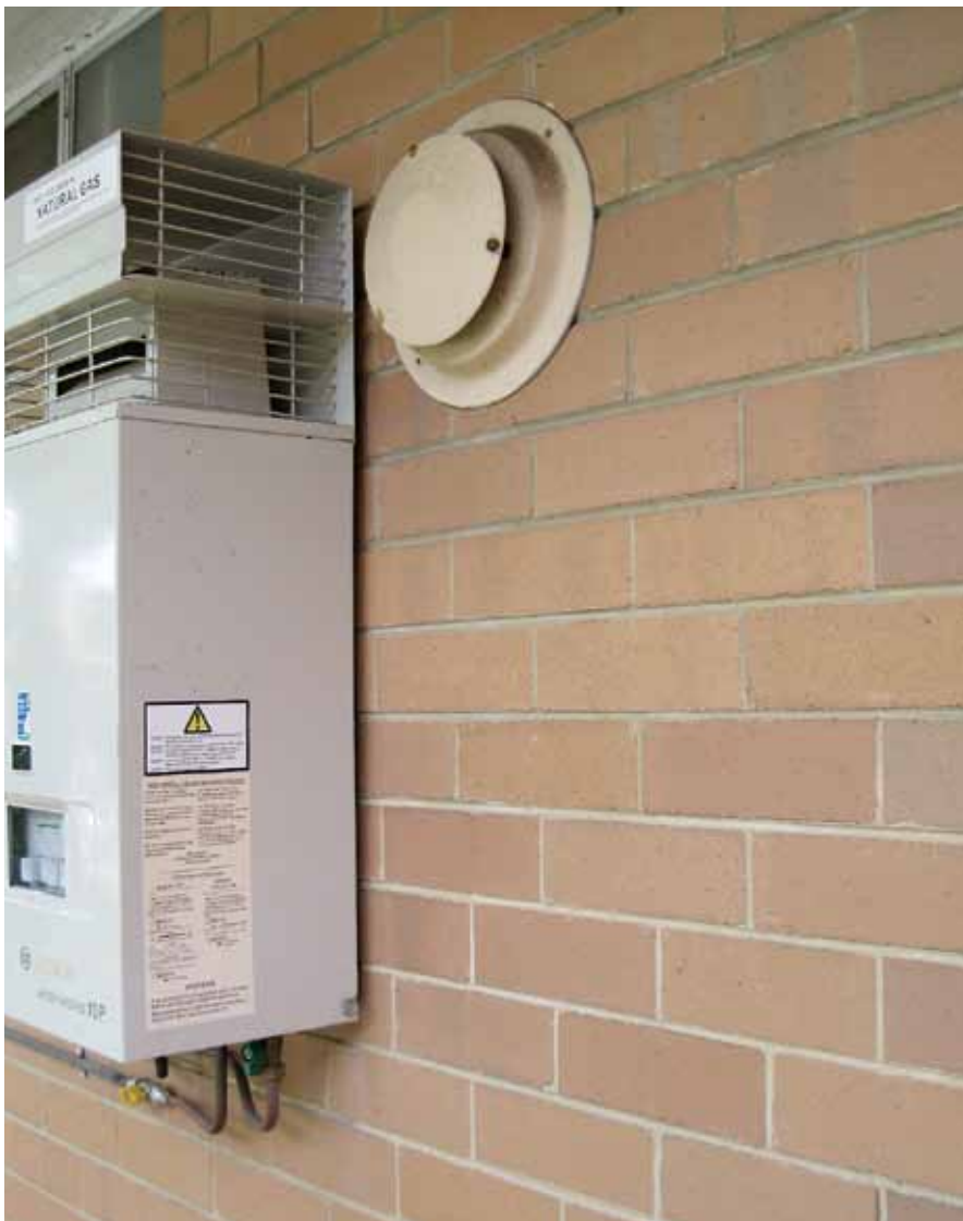
Gas water heater flue installed without adequate clearance from naturally ventilated exhaust cowl (opening)
