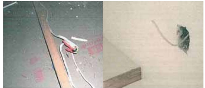
Cable junction in roof space not enclosed. Light switch cable which has not been terminated.
