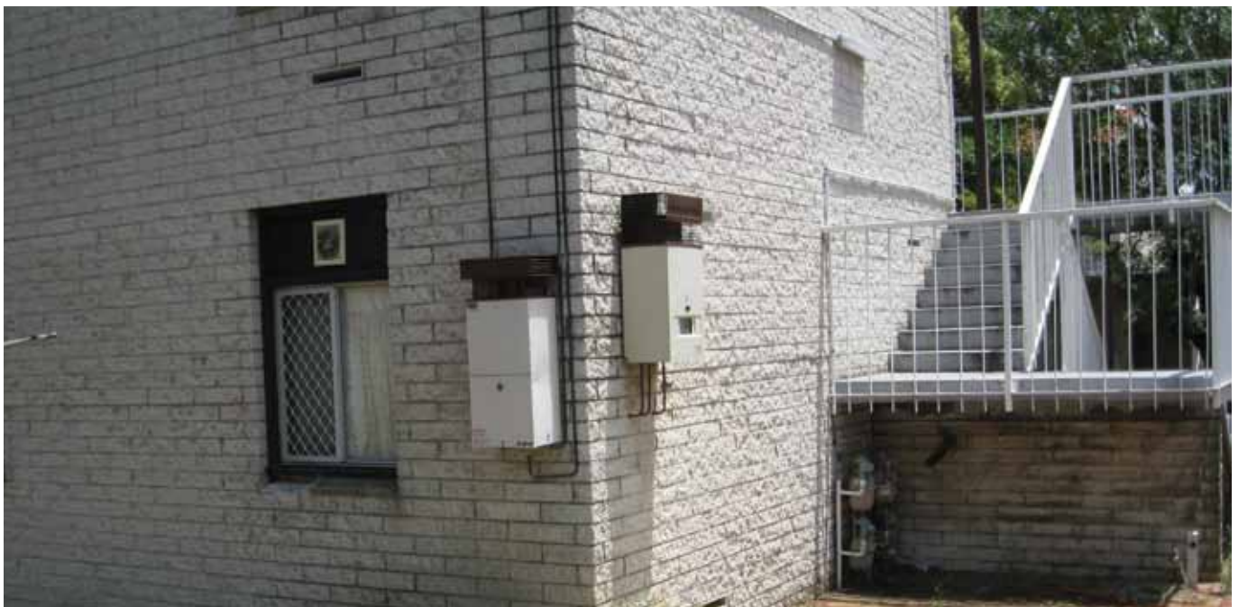
Gas water heaters installed with insufficient clearance from an external corner
