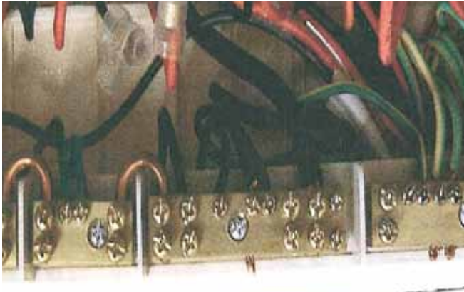
Distribution switchboard showing no MEN connection.
