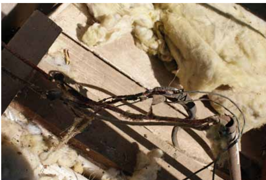
Deteriorated rubber insulation exposing live conductors.
