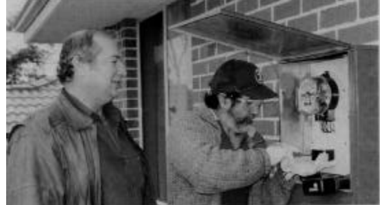
Peter Rowson of DBR Electrics oversees his electrician Renato Varricchio completing the first installation connected under the new Western Power connection arrangement
